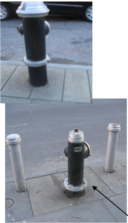
These two are examples of Fire Hydrants surrounding the whole are of Stuyvesant Square
