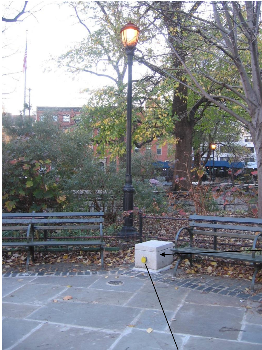
Water pipe, incase of emergency
