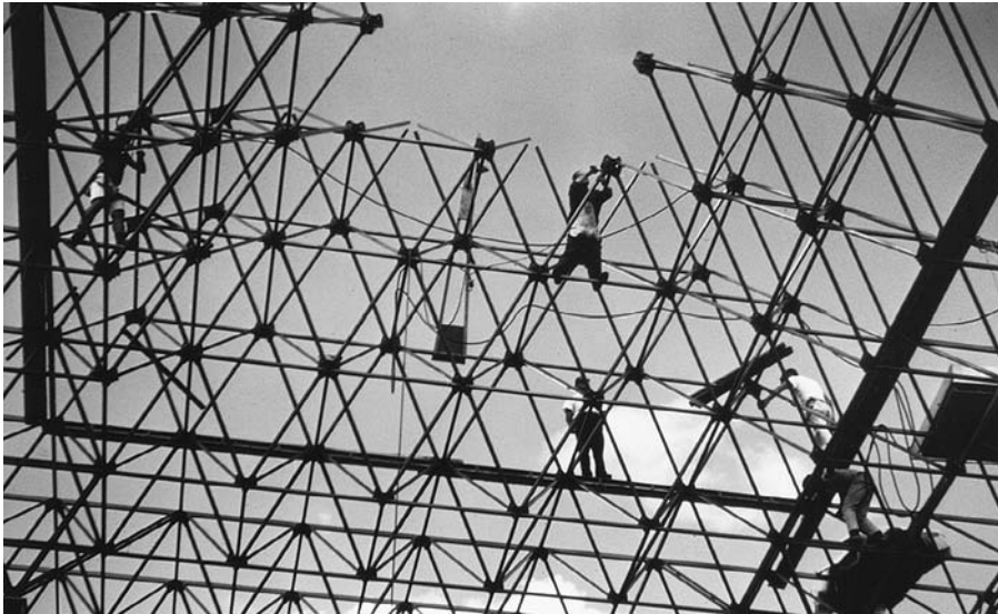
FIGURE 11.85 Assembling a space truss. (Courtesy of Unistrut Space-Frame Systems, GTE Products Corp.)
