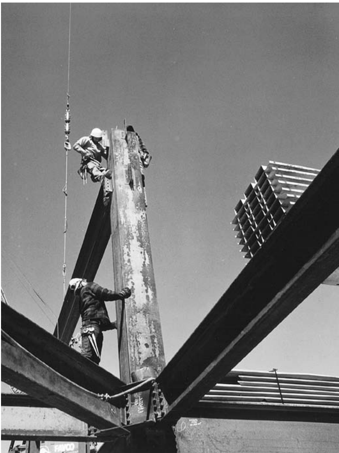
FIGURE 11.53 Ironworkers attach a girder to a box column. Each worker carries two combination wrench–drift pin tools in a holster on his belt and inserts the tapered drift pins into each connection to hold it until a few bolts can be added. Bundles of corrugated steel decking are ready to be opened and distributed over the beams to make a floor deck. (Courtesy of Bethlehem Steel Corporation)
