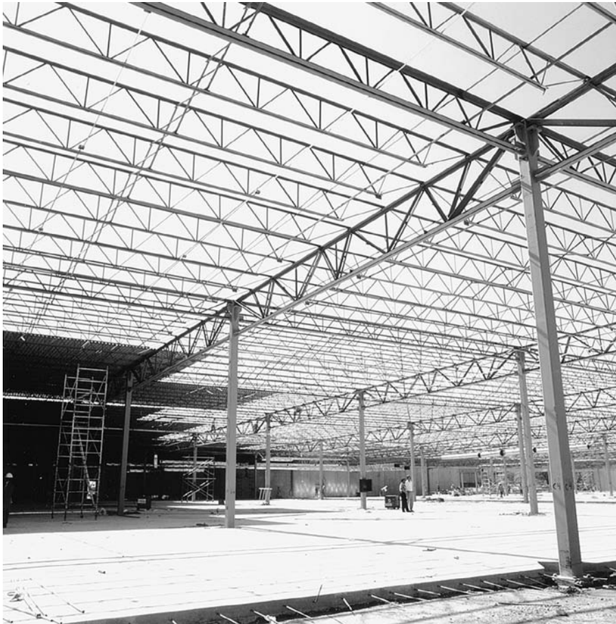
FIGURE 11.14 The roof of a single-story industrial building is framed with open-web steel joists supported by joist girders. The girders rest on columns of square hollow structural sections. (Courtesy Vulcraft Division of Nucor)
