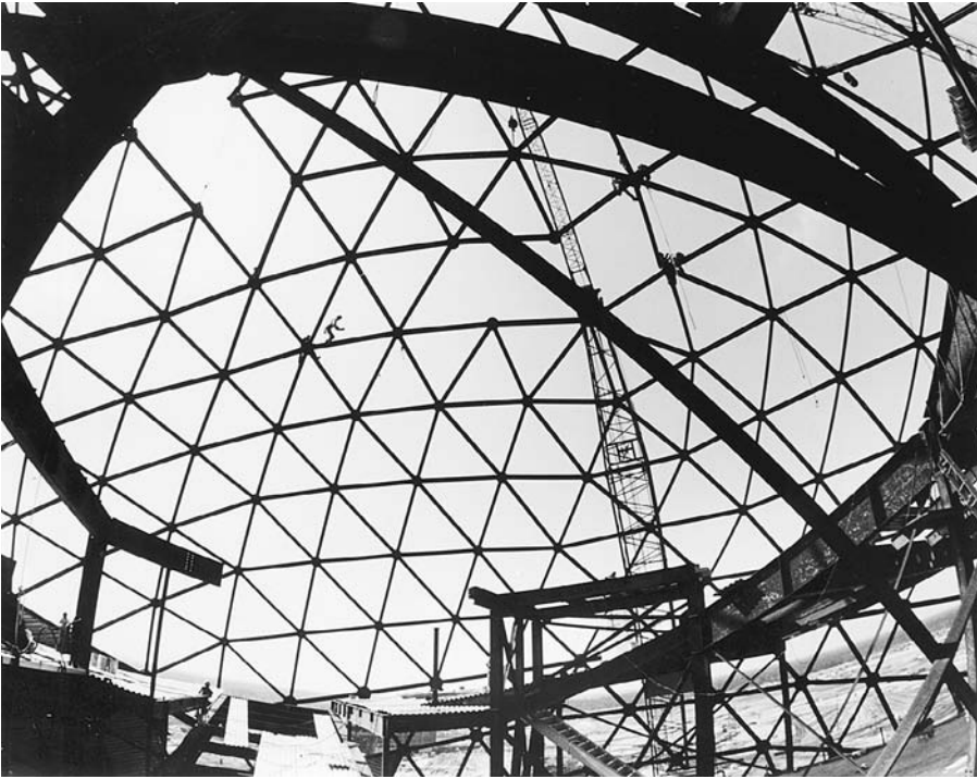
FIGURE 11.87 Erecting the steel dome at Disney World. (© Walt Disney Productions. Permission of American Institute of Steel Construction)
