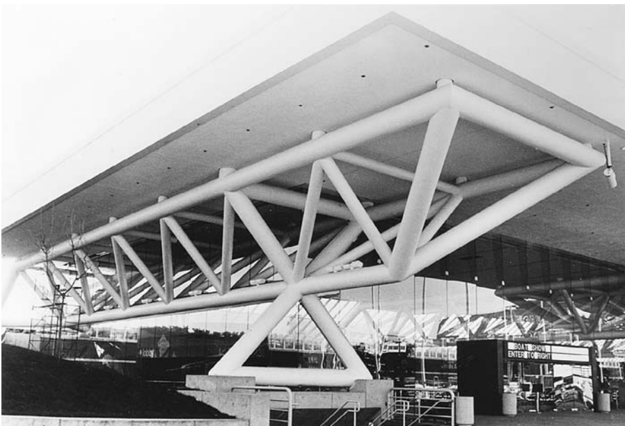
FIGURE 11.84 Tubular steel trusses support the roof of a convention center. (Permission of American Institute of Steel Construction)
