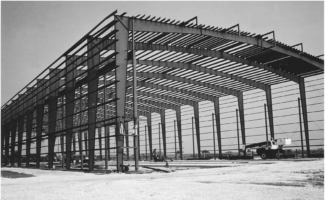
FIGURE 11.80 The steel rigid frames of this industrial building carry steel purlins that will support the roof deck and girts to support the wall cladding. The depth of each frame varies with the magnitude of the bending forces and is greatest at the eave connections, where these forces are at a maximum. (Courtesy of Metal Building Manufacturers Association)
