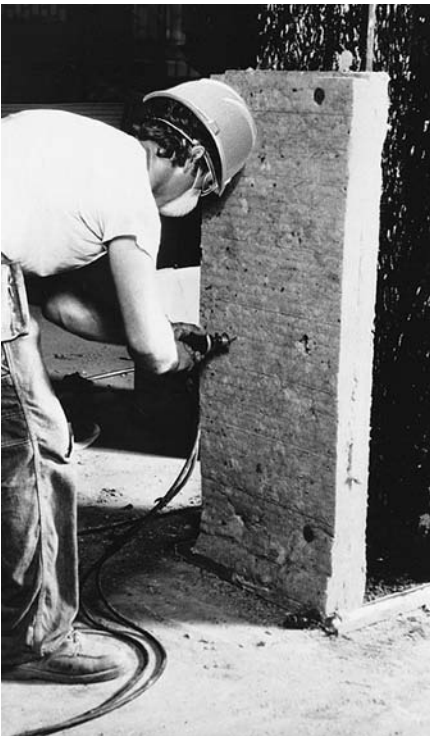
FIGURE 11.74 Attaching slab fireproofing made of mineral fiber to a steel column, using welded attachments. (Courtesy of United States Gypsum Company)
