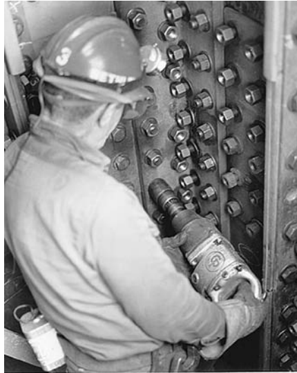
FIGURE 11.16 An ironworker tightens high-strength bolts with a pneumatic impact wrench. (Courtesy of Bethlehem Steel Corporation)
