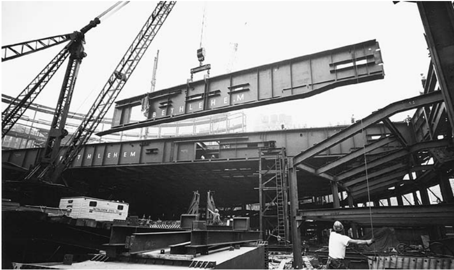
FIGURE 11.79 Erecting a welded steel plate girder. Notice how the girder is custom made with cutouts for the passage of pipes and ductwork. The section being erected is 115 feet (35 m) long, 13 feet (4 m) deep, and weighs 192,000 pounds (87,000 kg). (Courtesy of Bethlehem Steel Corporation)
