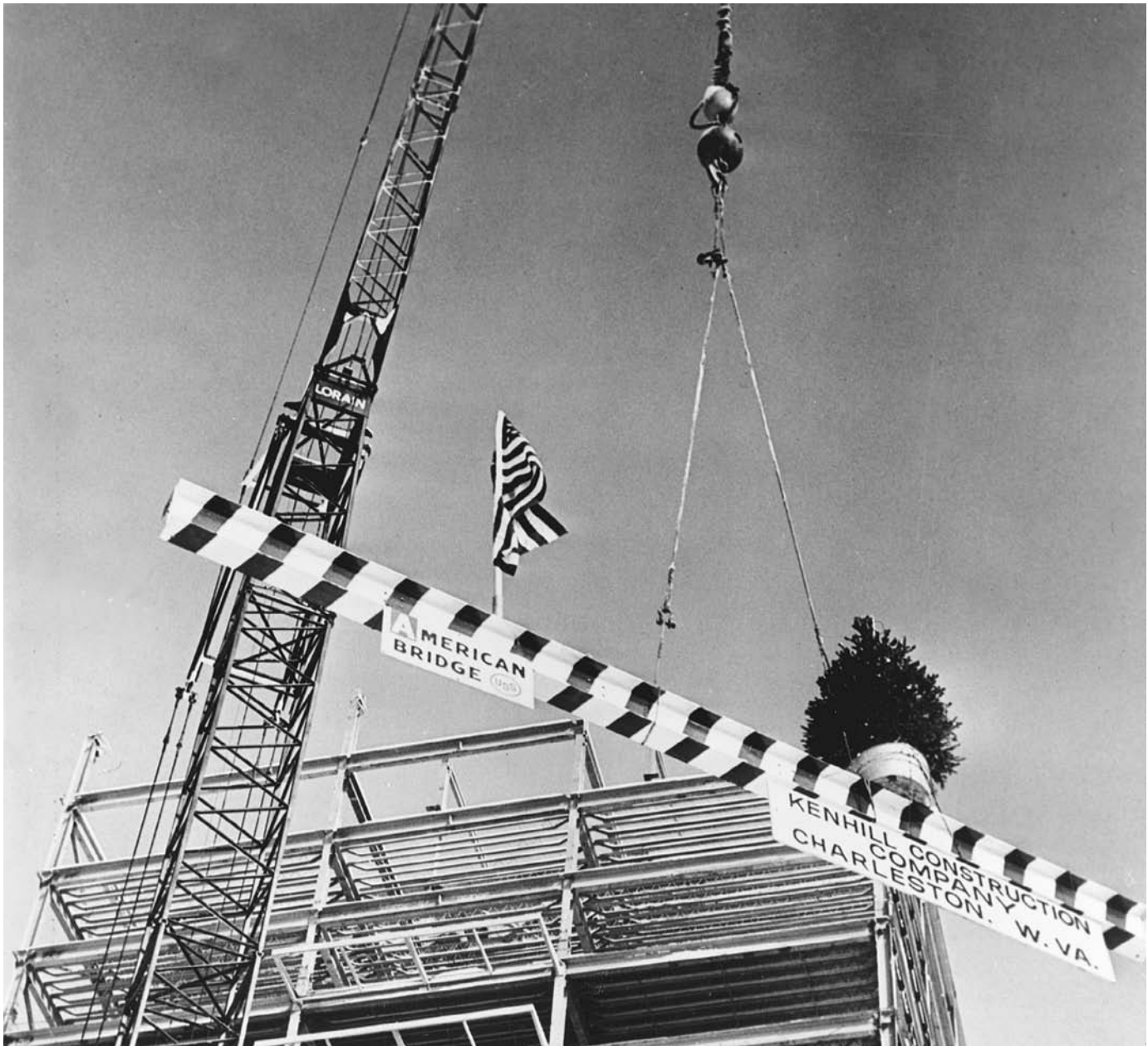
FIGURE 11.56 Topping out: The last beam in a steel frame is special. (Courtesy of U.S. Steel Corp.)
