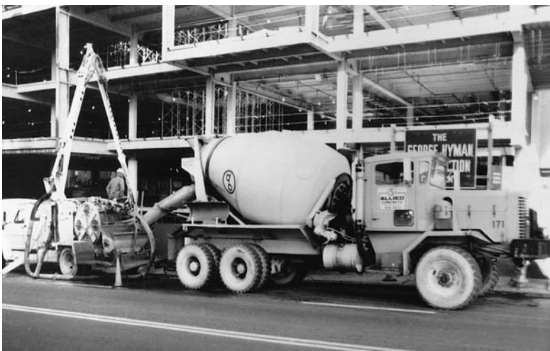
FIGURE 13.10 A transit-mix truck discharges its concrete, which was mixed en route in the rotating drum, into a truck-mounted concrete pump, which forces it through a hose to the point in the building at which it is being poured. (Reprinted with permission of the Portland Cement Association from Design and Control of Concrete Mixtures, 12th edition; Photos: Portland Cement Association, Skokie, IL)
