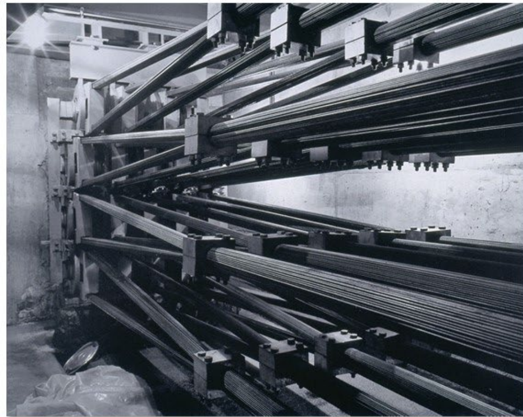
Photograph inside the anchorage showing the 19 steel wire strands splitting to 38 strands to loop around the cast iron shoes
