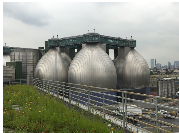
The wastewater treatment plant at work.
