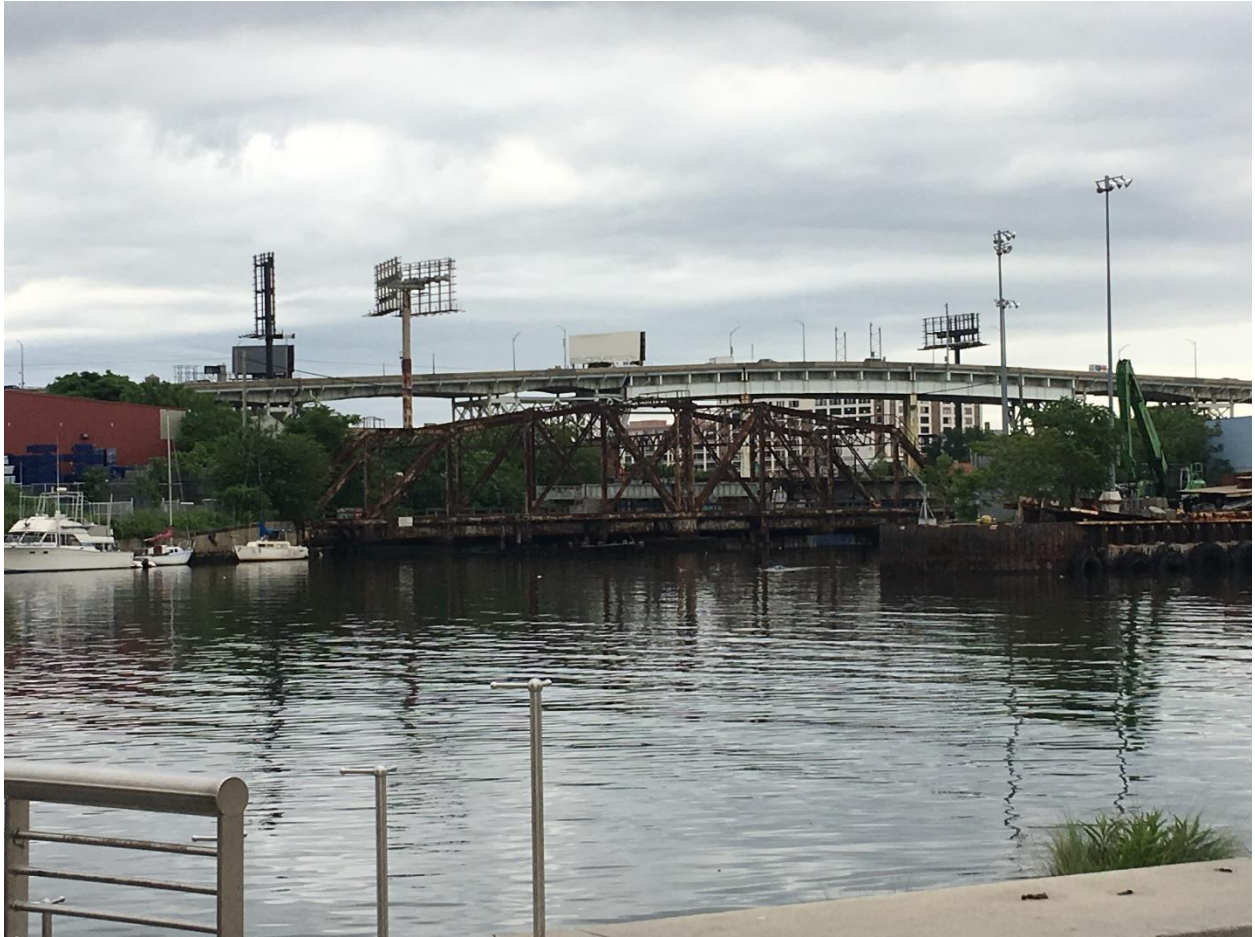
The rust frozen bridge
