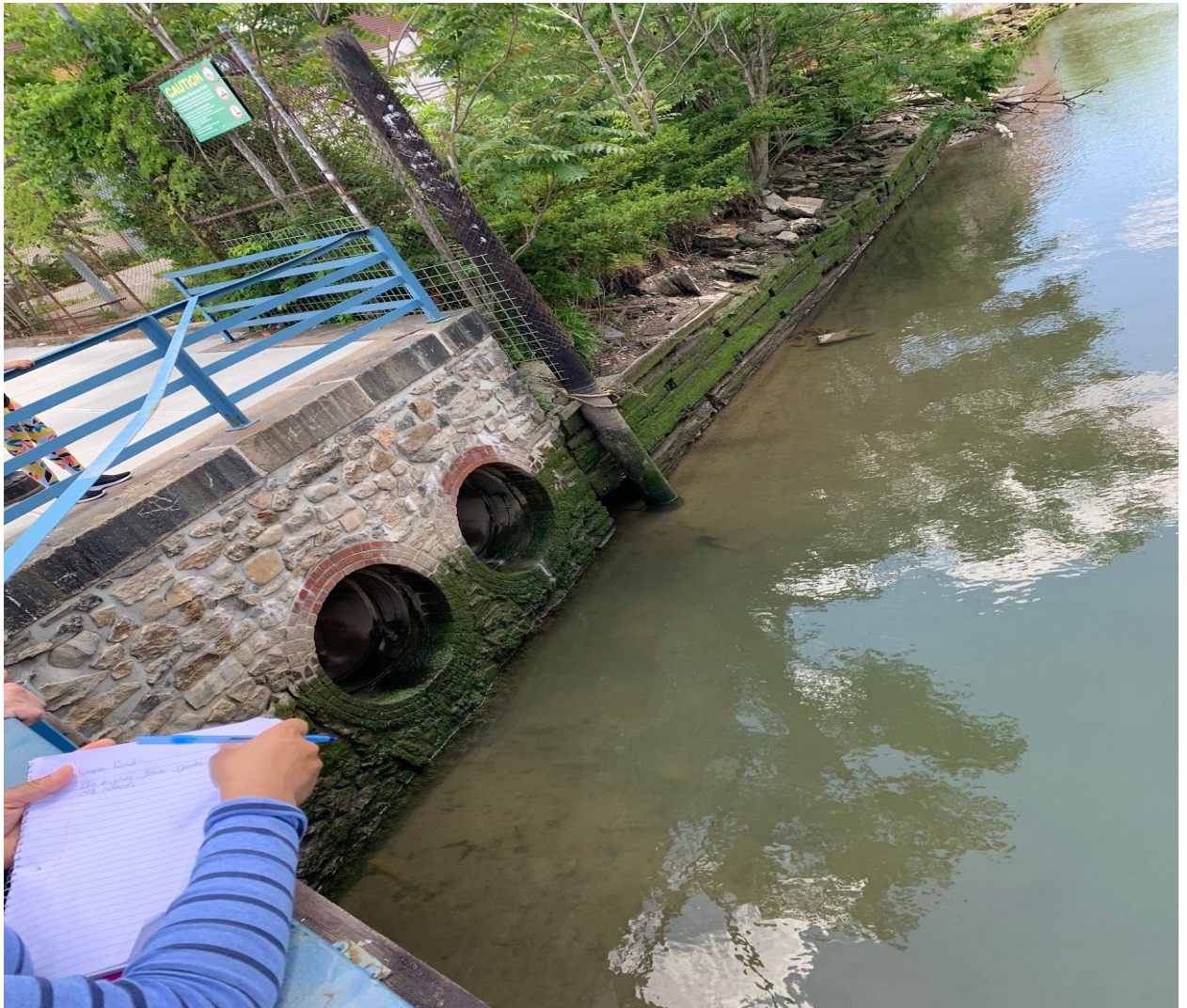
Sewage Pipes leading to Gowanus
