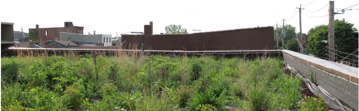
Native Meadow Rooftop Garden, Linda Tool and Die, Red Hook (image © 2010 John Seitz )
