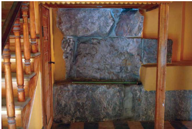
Figure 14 Three courses of ashlars in the hallway between the third courtyard and service courtyard (G. H. Lewis).
