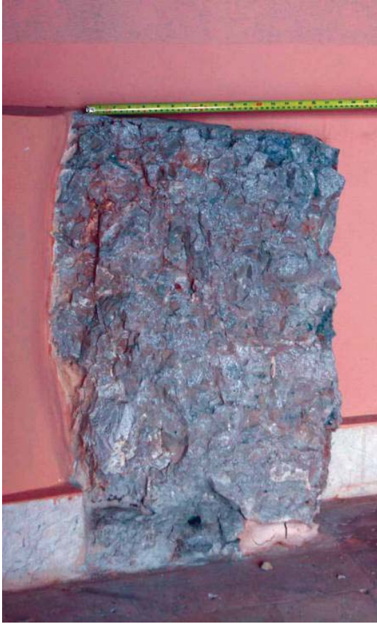
Figure 17 Detail, northern section of the Roman wall in Fig. 13, the south-eastern bedroom, the service courtyard (G. H. Lewis).
