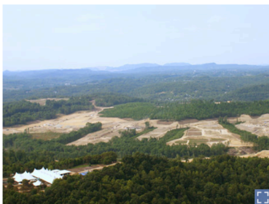
The Summit Bechtel Family National Scout Reserve while under construction in 2011. The camp will open in July 2013 with the National Scout Jamboree.
