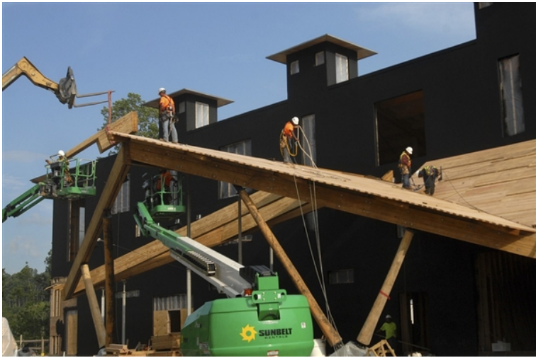
Craig Cunningham / Charleston Daily Mail A construction crew works on the welcome center at Summit Bechtel Family National Scout Reserve in Glen Jean, W. Va. Some 40,000 Scouts, leaders and others will descend on southern West Virginia for the first National Scout Jamboree at the site next week.
