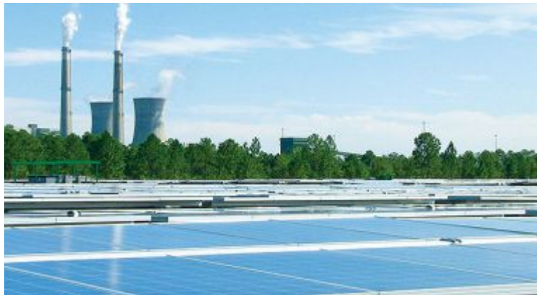
Solar panels at Curtis H. Stanton Energy Center. Photo by OUC Reliable One/Wikimedia Commons
