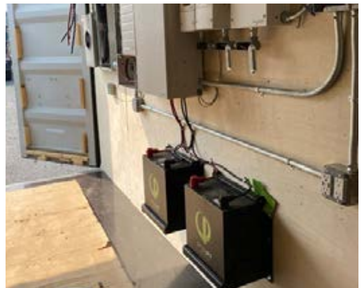
City Tech CSC Solar+Storage Training Lab, BNYDC
