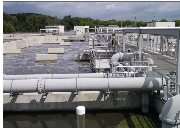
Altoona Water Authority, Easterly WWTF
