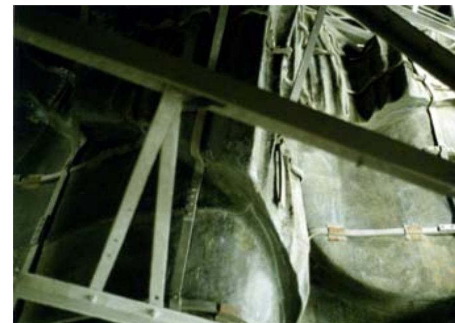
Stainless steel armatures attached to the copper sheets of Liberty's skin link to an iron scaffolding ( www.statuecruises.com )
