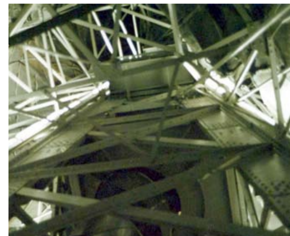
An iron pylon serves as the Statue of Liberty's core. This framework also supports a spiral staircase that winds up through the structure.
