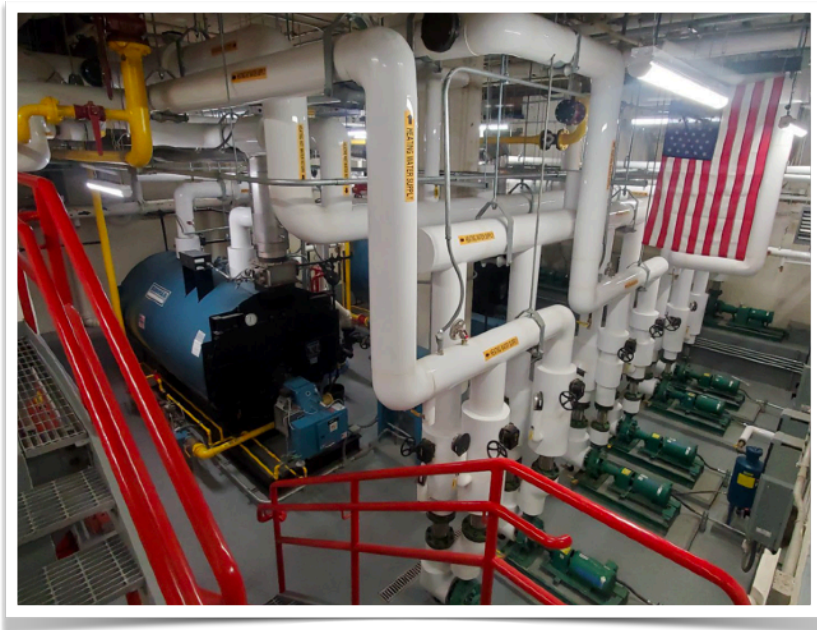
Voorhees Mechanical Room Upgrade was completed last year as part of Phase I Renovations.
