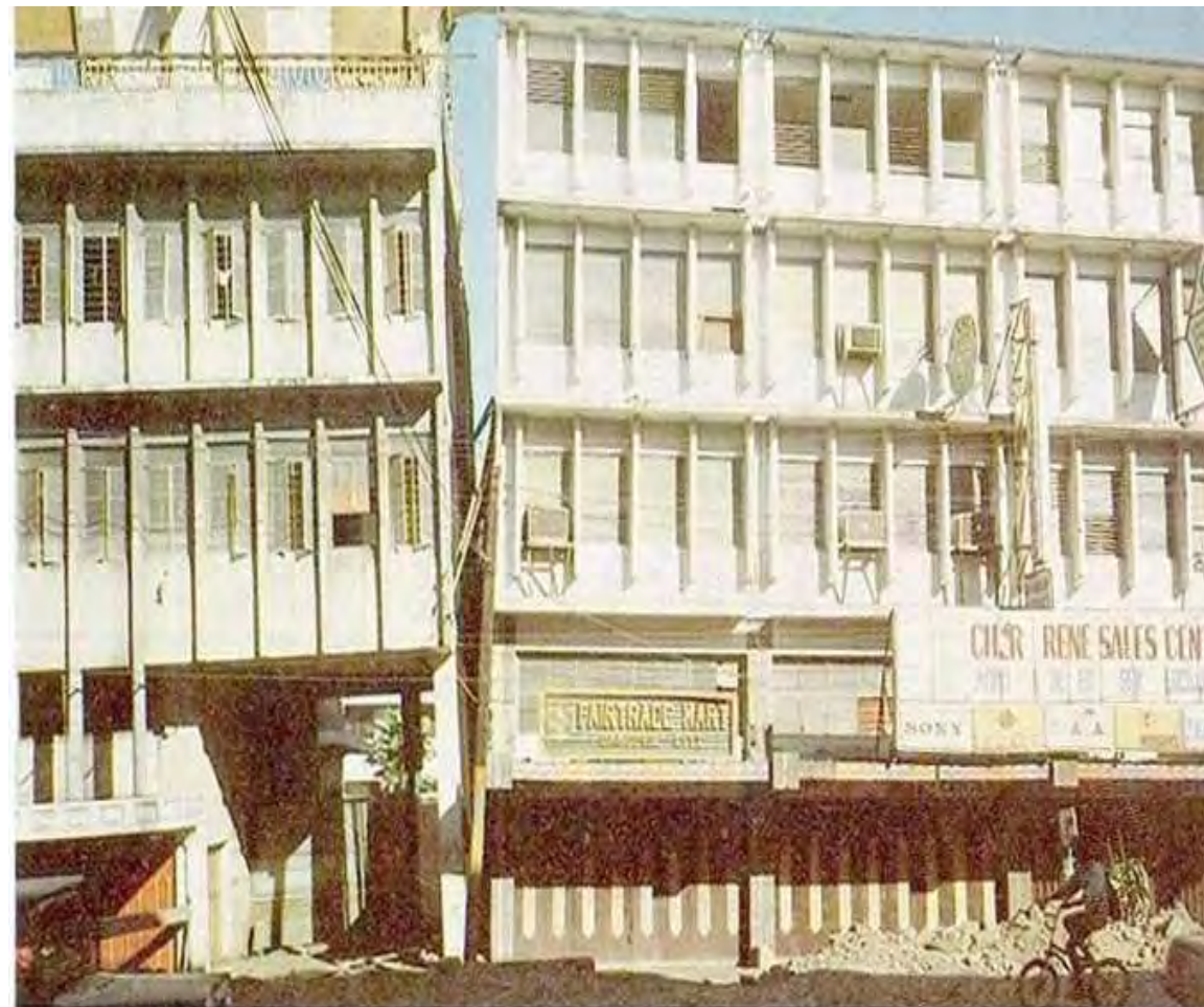
Uneven sinking and tilting on Fernandez Avenue (G. Rantucci)
