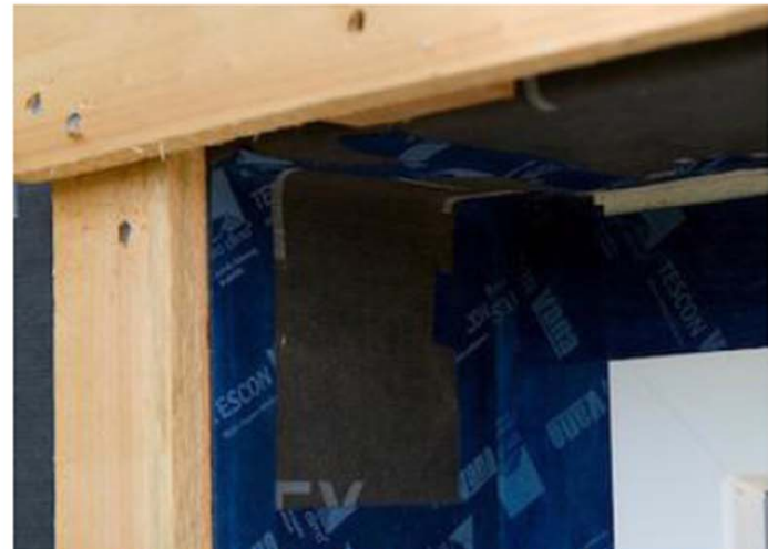
Exterior window with SOLITEX Mento Plus wrapped into rough opening. Taped connections include membrane seams (TESCON Vana) and window frame connections (TESCON Profil).
