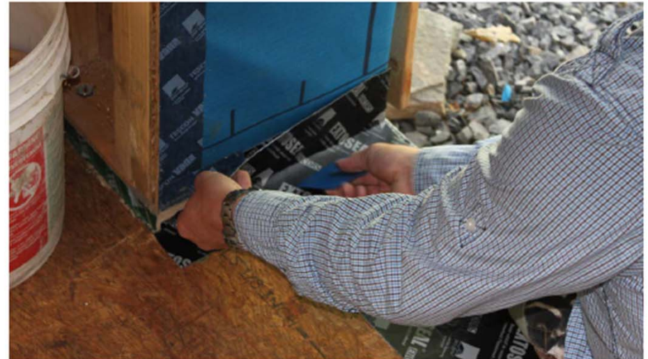
Applying EXTOSEAL Encors and EXTOSEAL Finoc at floor-to-ceiling window (or door). Finoc is used as a capillary break at wall to floor connections. Encors is a self-sealing sill tape for watertight screw/nail penetrations.
