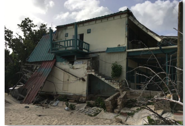
↑ Damage assessment tour on St. Thomas
