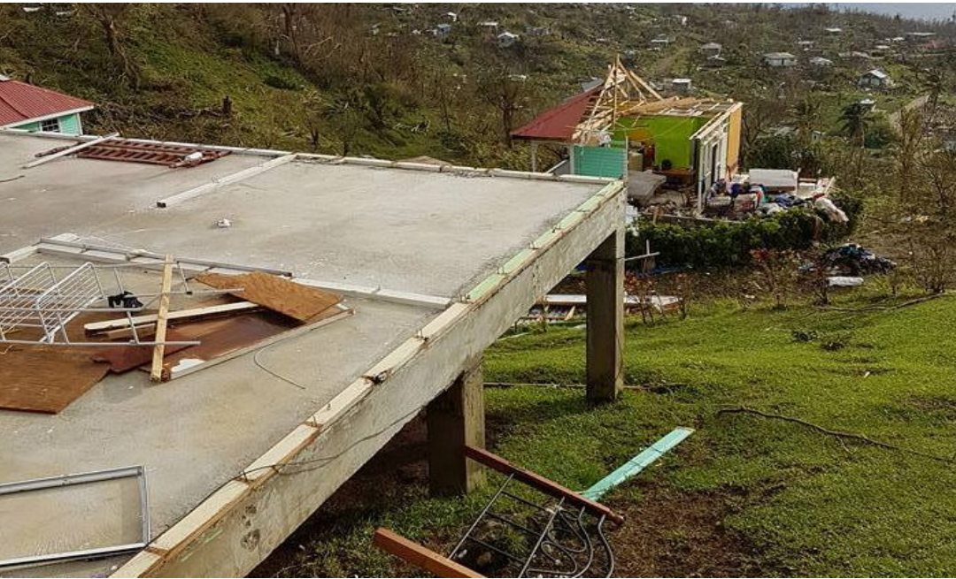
(2) Former house damaged by Hurricane Maria
